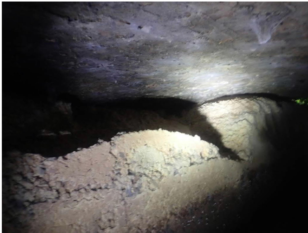
Photo 12 shows an area of damage to the top of the right abutment
