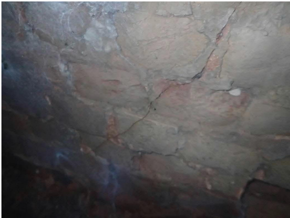
Photo 14 shows a crack to the soffit at 4.7m
