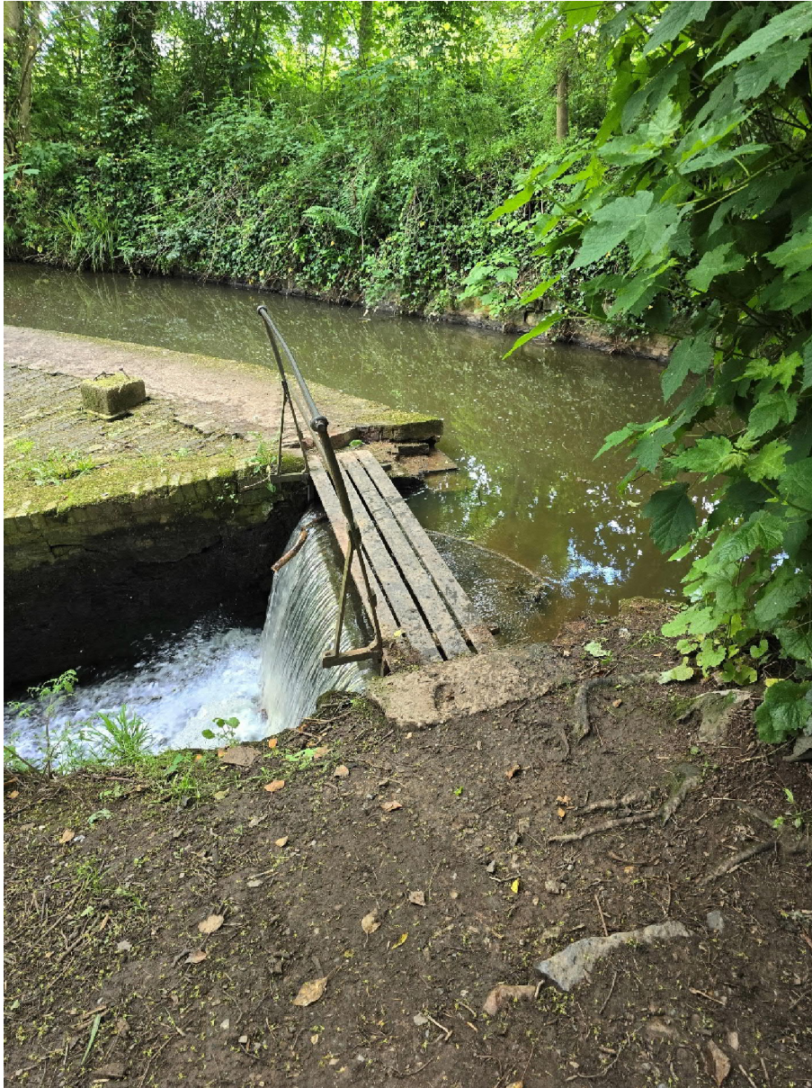
Non-compliant foot bridge to north of subject bridge.
