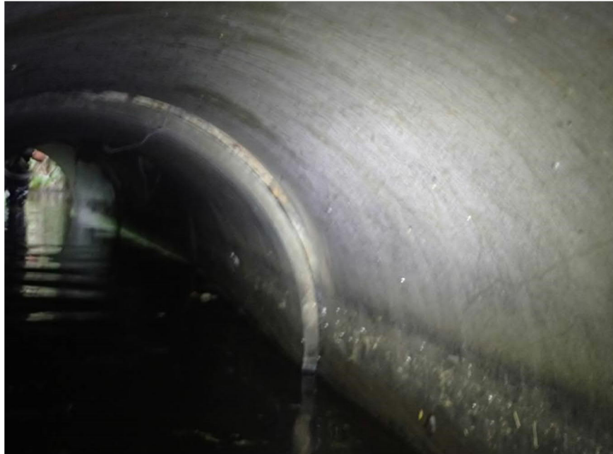
Figure 10: Photo extract from 2017 inspection report showing pipe defects.
