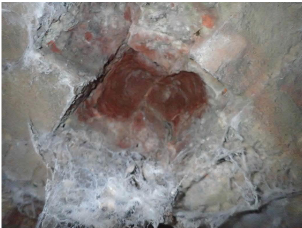
Photo 13 shows a void to the soffit at 2.4m
