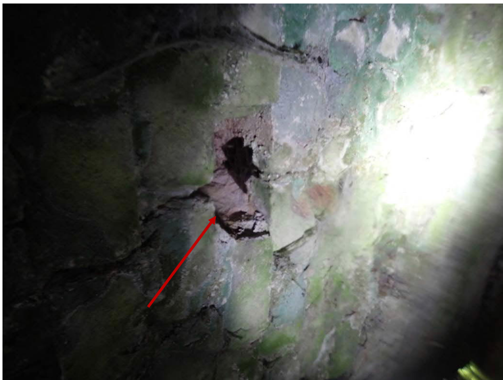
Photo 3 shows an area of missing stonework at 0.3m
