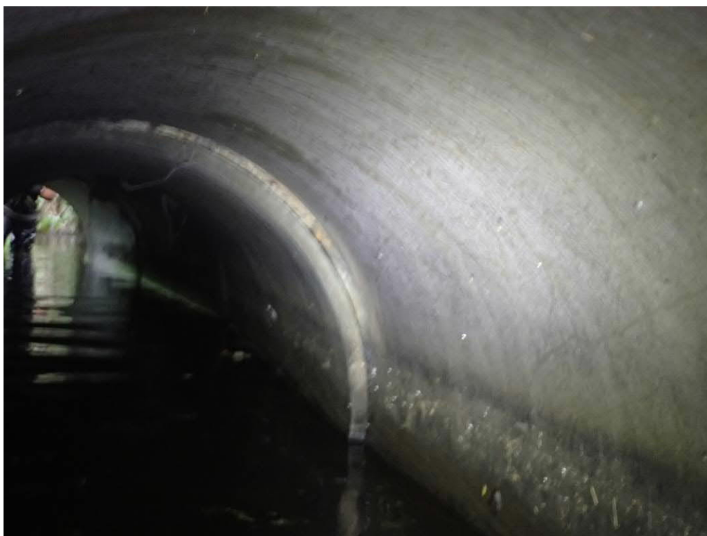
Photo 9 shows misalignment to a joint section at 5.1m
