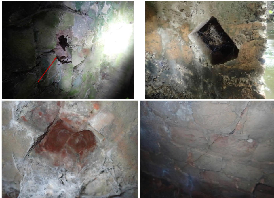
Figure 9: extracts of photos from 2017 inspection report showing bridge soffit defects.
