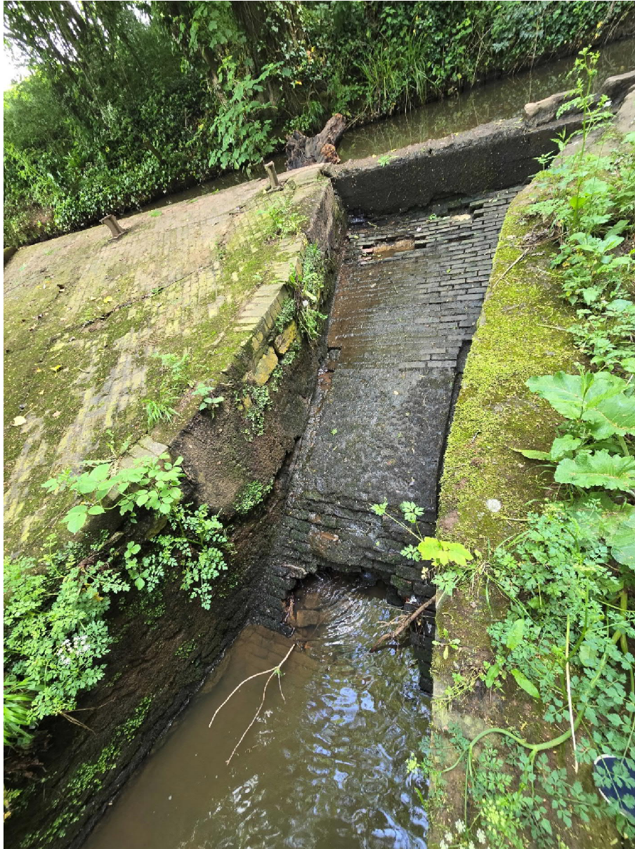
Defective spillway to north of bridge.
