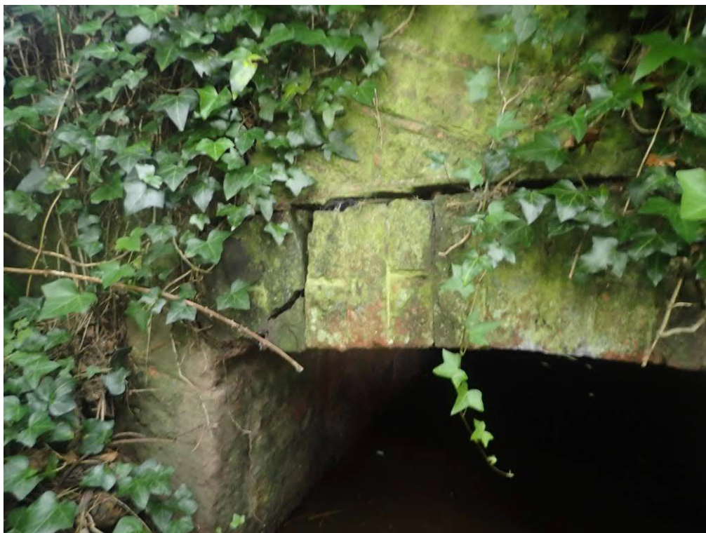
Photo 7 shows a crack to the arch masonry at the inlet
