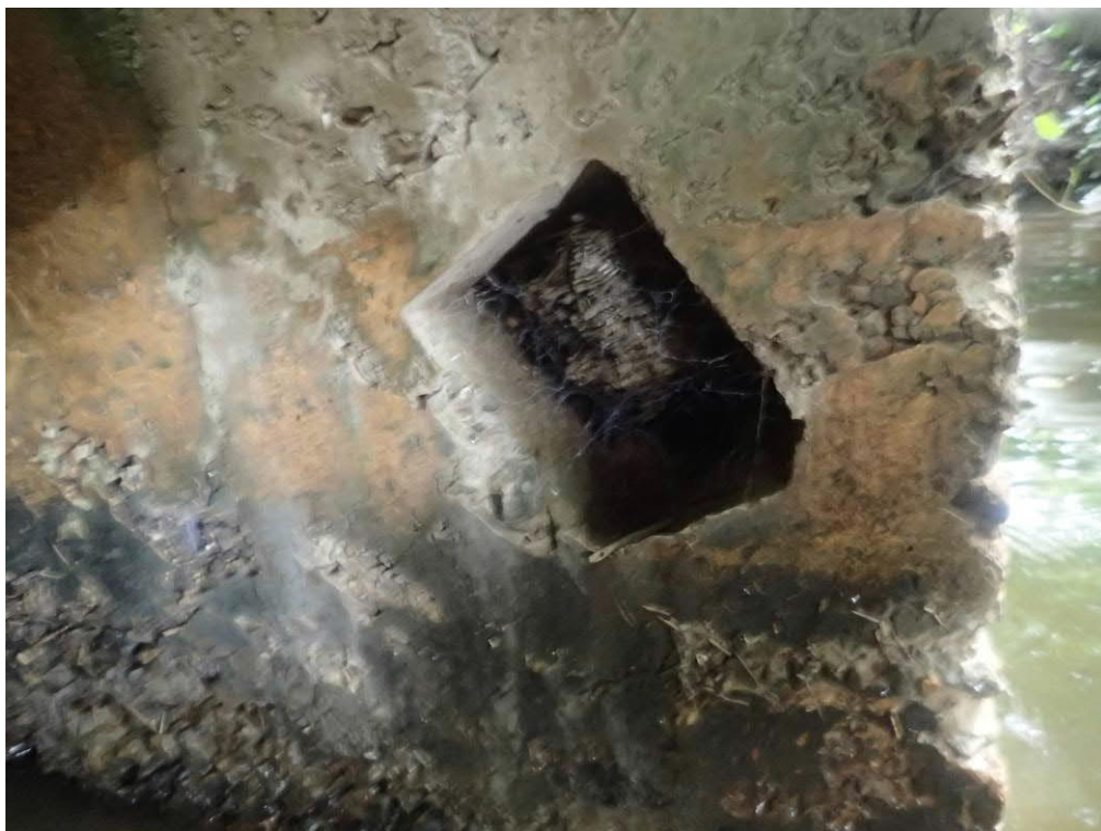
Photo 5 shows a void to the left abutment at 9.2m
