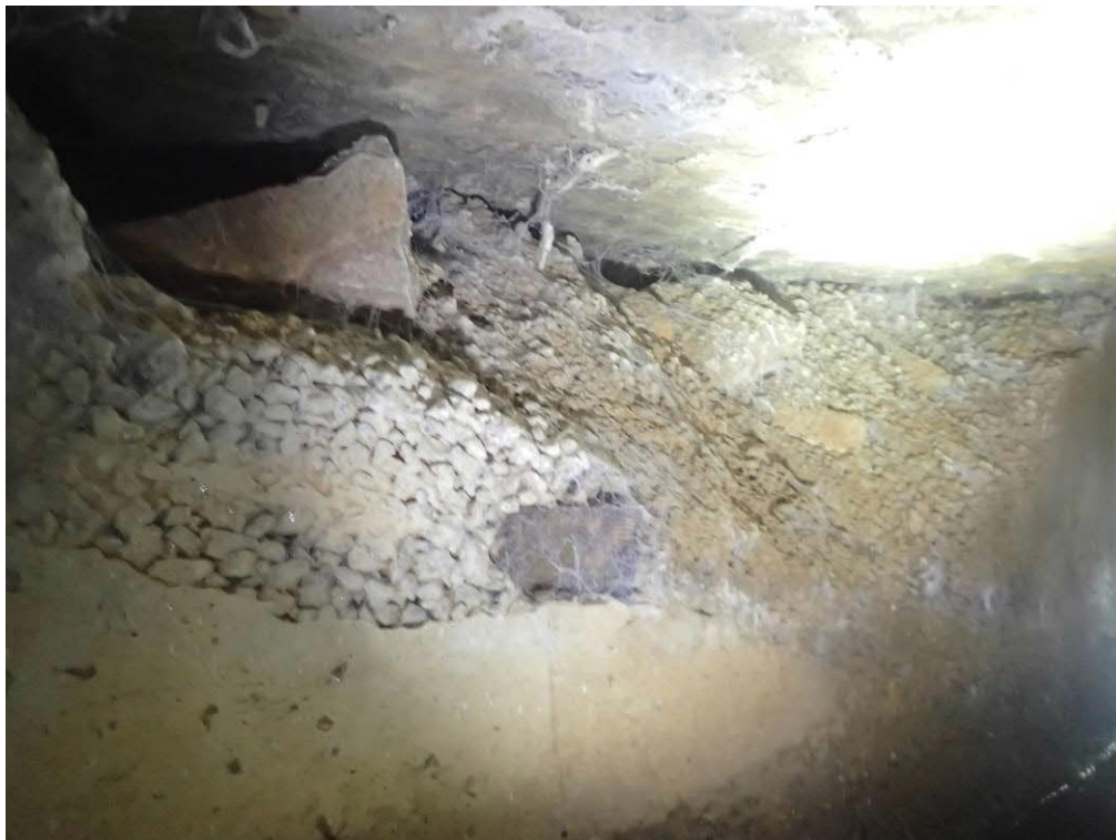
Photo 4 shows an area of damage to the top of the left abutment at 5.7m
